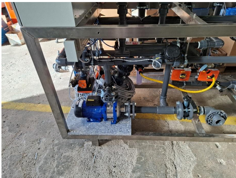
RECYCLED FRC PANEL USED AS PLATFORM FOR A WATER PUMP
