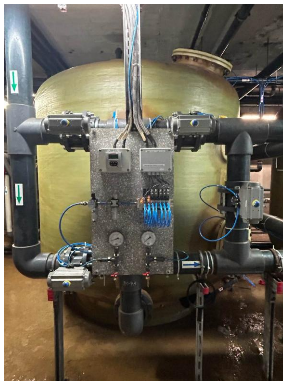
PANEL INSTALATION IN PUBLIC POOL MACHINE ROOM
